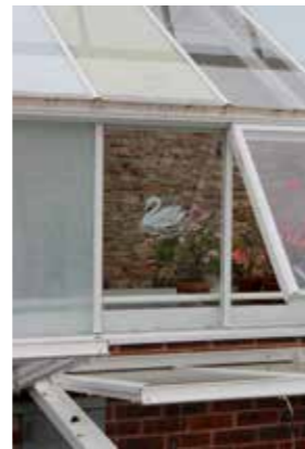
The Bishop's Palace greenhouse with opaque Doultling Stone and Swan White on roof panels. Vertical window panes painted with translucent White Witch & Swan White stencil designs
