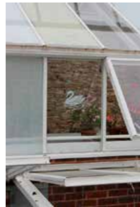
The Bishop's Palace greenhouse with opaque Doultong Stone and Swan White on roof panels. Vertical window panes painted with translucent White Witch & Swan White stencil designs
